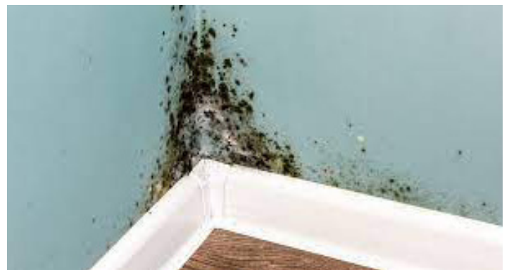
Mould can look like this
